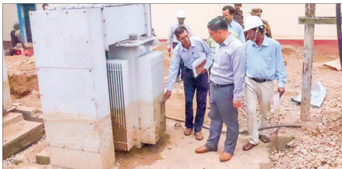
Kayah State Chief Minister U Zaw Myo Tin looks into the ongoing restoration work inside the No 2 Biluchaung Hydropower Plant (Lawpita) yesterday. PHOTO: KAYAH STATE IPRD
