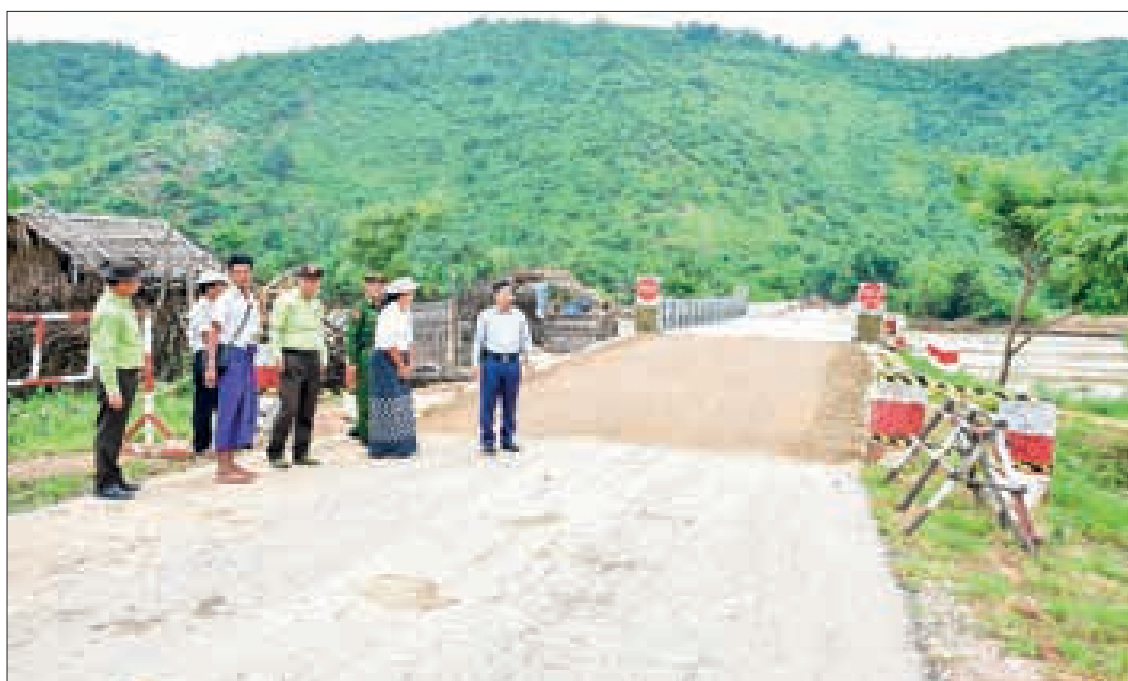
Nay Pyi Taw Council Chairman U Than Tun Oo looks into the construction of a 80-foot two-layer temporary bailey bridge yesterday at the site of Zeephyupin Village bridge across the Paunglaung River damaged by water erosion.
