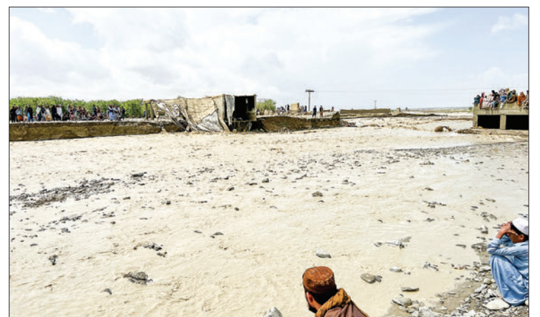
Residents gather beside a collapsed bridge due to flood waters following heavy rains in Pishin district on 15 April 2024. PHOTO: AFP
