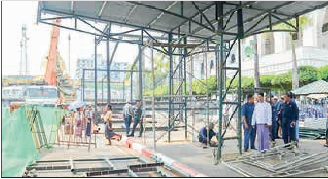
The photo shows the construction work of the Yangon City Hall Central Pavilion and water-splashing pandals on 15 March.
