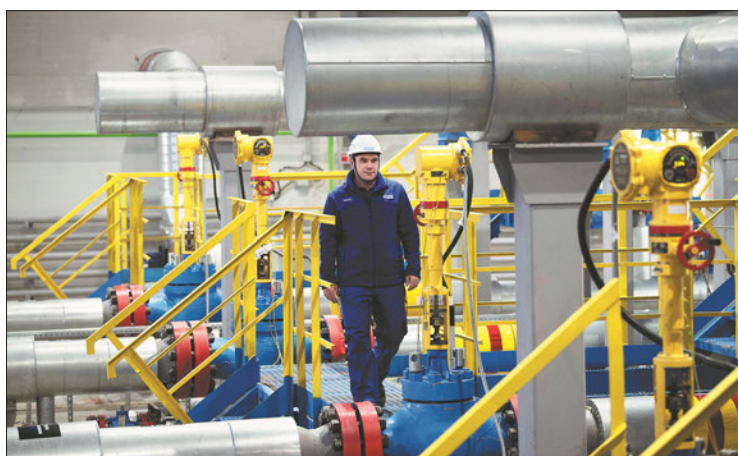
A worker patrols the Kovykta natural gas field in Russia's Irkutsk region in December, days before the gas field began operations on 20 March 2023. PHOTO: XINHUA/FILE
