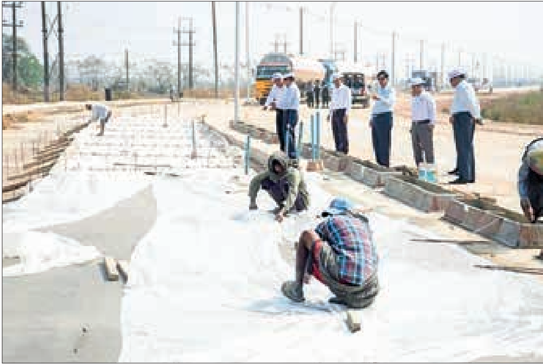
The photo shows Yangon Region Chief Minister U Soe Thein is observing the expansion of the frontage road of the Thilawa Port and establishing the lamp-posts along the traffic island.
