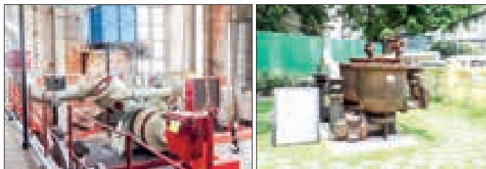
The photo depicts coal-fired boiler blowers and electric-powered boiler blowers.
