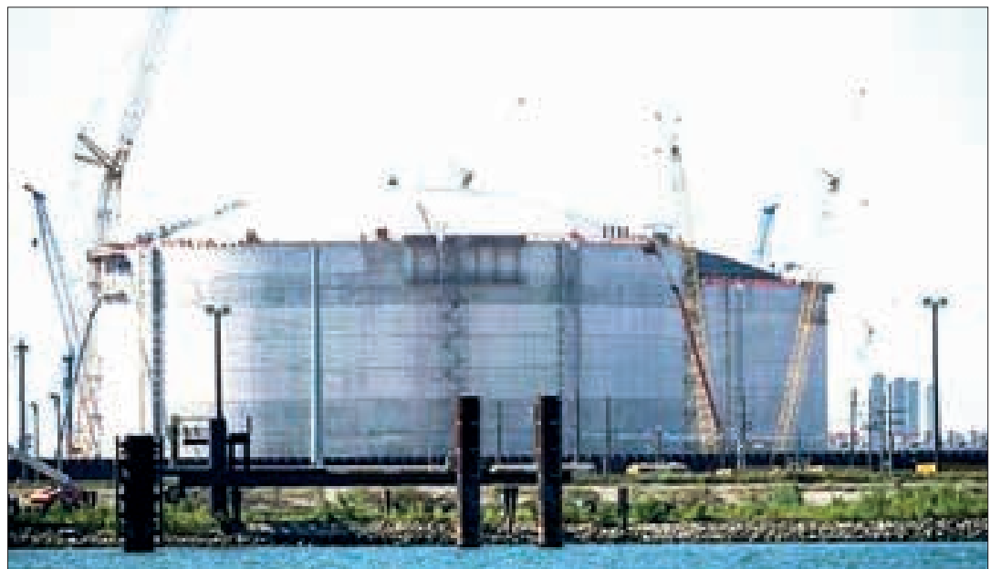
Cranes are seen near the construction site of the Venture Global LNG plant next to the Mississippi River in Plaquemines Parish south of New Orleans, Louisiana. PHOTO: AFP
