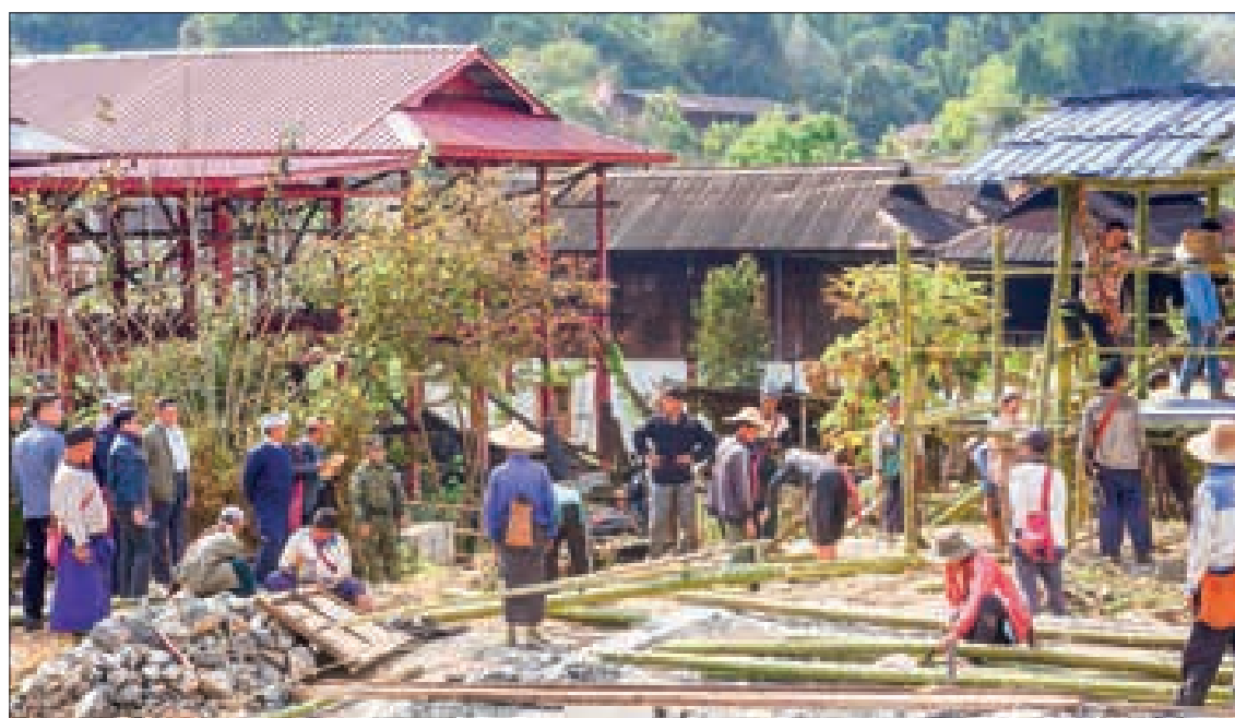
SAC Member Khun San Lwin views the house reconstruction site in the Pa-O Self-Administered Zone yesterday.
