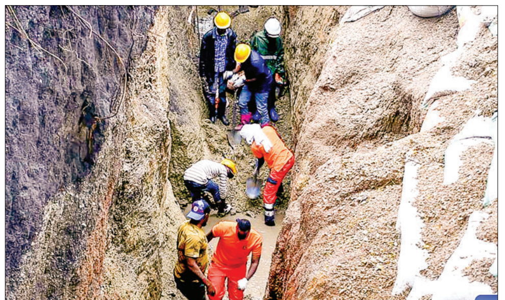
Rescuers search for survivors at a gold mine after it collapsed following a heavy downpour in Simiyu region, Tanzania, 14 January 2024. Tanzanian authorities on Sunday closed down mining activities at a gold mine that killed 22 miners after it had collapsed on Saturday morning in Simiyu region in northern Tanzania. PHOTO: XINHUA
