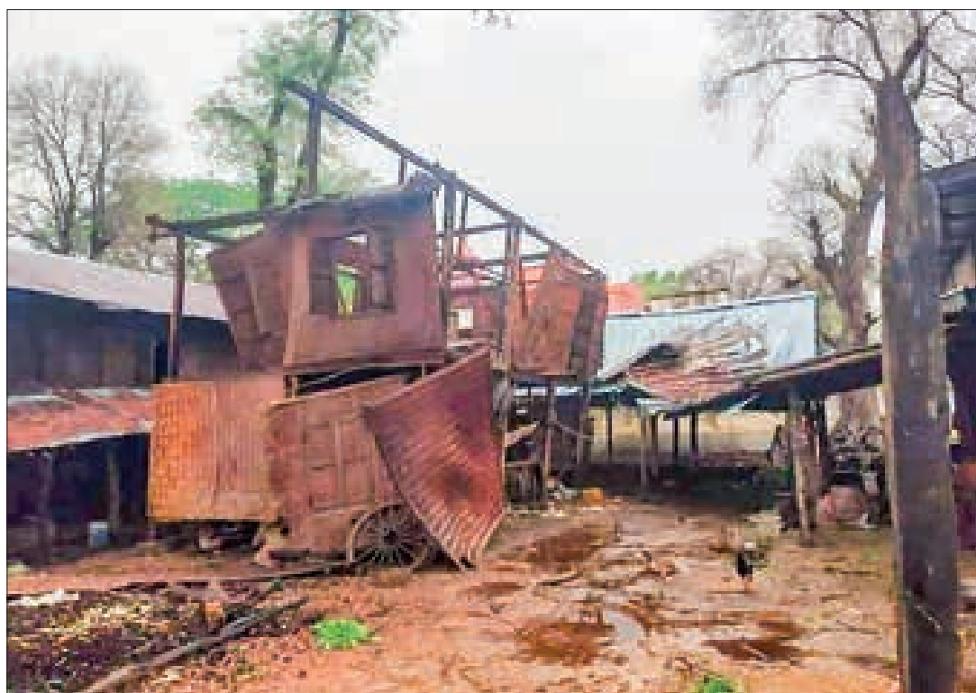
A house was damaged by strong wind on 21 April 2023 at Thamonkon village located in Natmawk township, Magway region.
