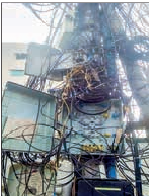
A glimpse of illegally connected fibres and Wi-Fi cables.
