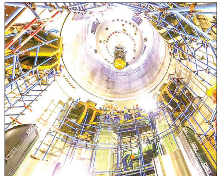
The first reactor pressure vessel of Shidaowan high temperature gas-cooled reactor nuclear power plant is hoisted in place on 20 March 2016. PHOTO: MA YUEJUN/XINHUA
