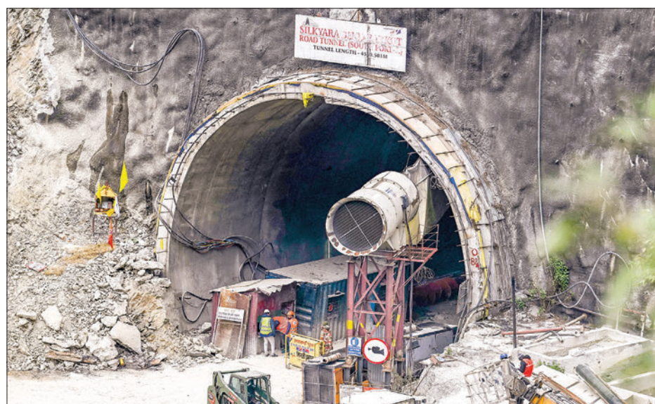
Rescue personnel work at the collapsed under construction Silkyara tunnel in the Uttarkashi district of India's Uttarakhand state, on 27 November 2023. PHOTO: AFP
