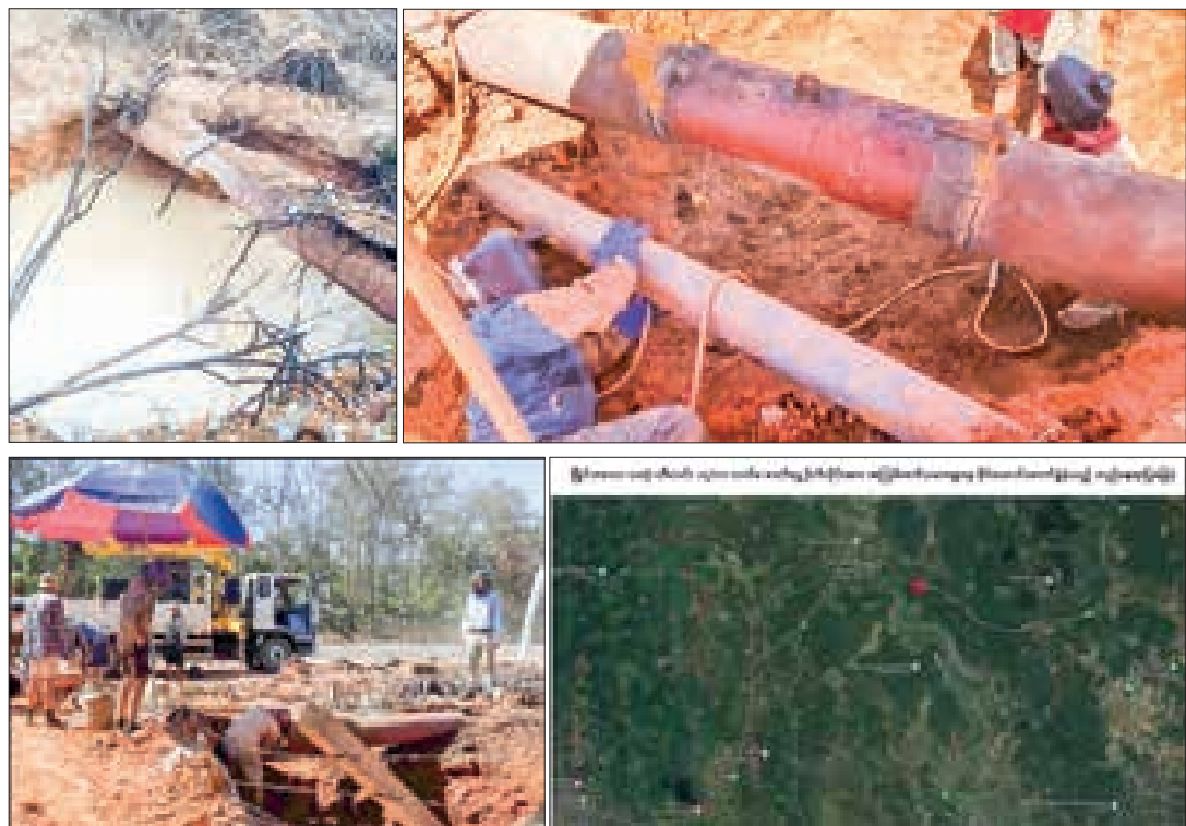
Photos show damage of the crude oil pipeline exploded by terrorists and preparations of the pipeline by officials of MOGE.
