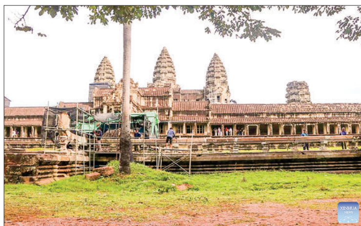
This undated photo shows the restoration site of a sandstone Naga balustrade at the southern side of the famed Angkor Wat temple in Siem Reap province, Cambodia. PHOTO: XINHUA
