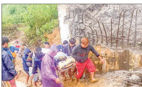
Security Forces clear and restore PyinOoLwin-Nawngkhio-Kyaukme-Lashio Union Highway for smooth public transport
