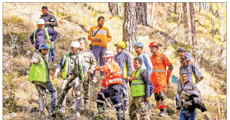
Independent disaster investigator Arnold Dix (C), President of the International Tunnelling and Underground Space Association and rescue workers conduct a survey at the Silkyara under construction road tunnel, days after it collapsed in the Uttarkashi district of India's Uttarakhand state on 20 November 2023. Indian rescuers were battling on 20 November, to free 41 men trapped in a road tunnel for nine days, as they prepared to dig an entirely new shaft after previous efforts failed. PHOTO: AFP
