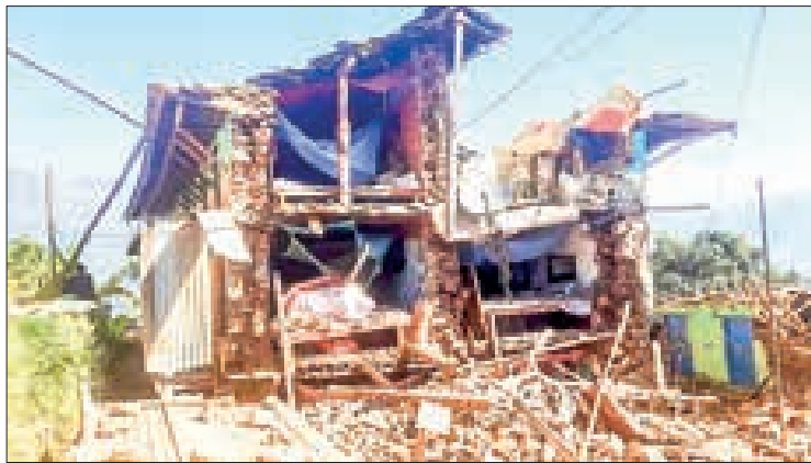
Damaged houses lie in ruins, in the aftermath of an earthquake at Pipaldanda village of Jajarkot district on 4 November 2023. PHOTO: AFP
