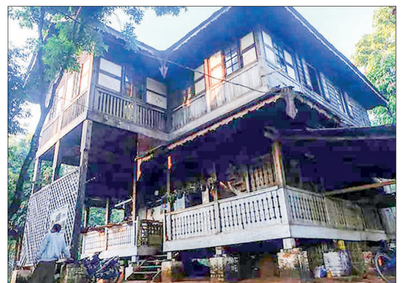
The photo shows the Tower House of Mr Maraе who was a Dolson ship company owner from colonial times.
