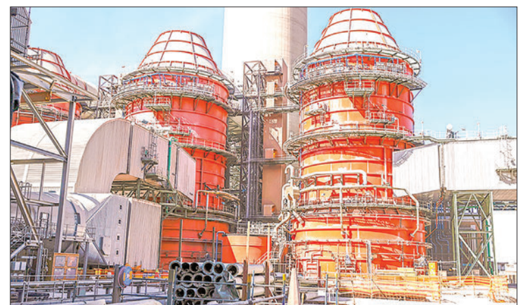
A general view of absorbers at the Kusile Power Station, a coal-fired power plant located on the Hartbeesfontein Farm in eMalahleni. PHOTO: AFP
