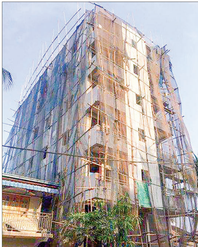
A building under construction in the municipal area of the Yangon City Development Committee.
