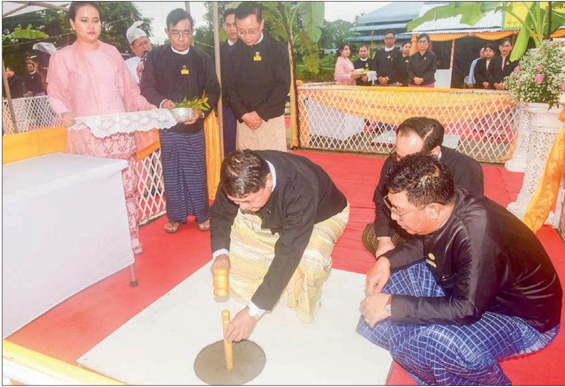
Chief Justice of the Union U Thar Htay drives the stake for new Insein District Court building, Insein Township, Yangon Region yesterday.
