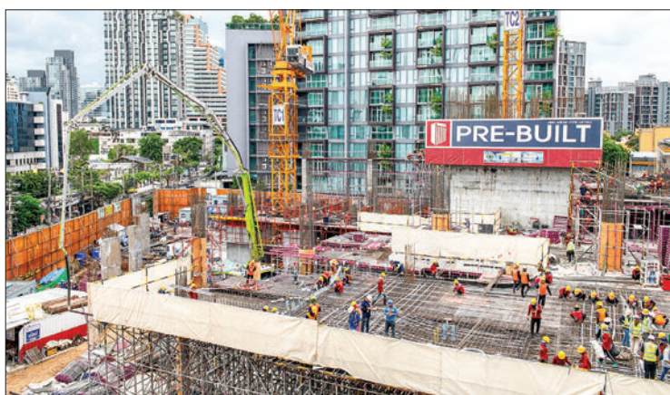
(FILES) Builders work at a construction site for a mixed-use development project in the Sukhumvit area of Bangkok on 1 July 2023. Thailand registered lower than expected economic growth of 1.8 per cent in the second quarter of 2023, official data released on 21 August 2023 showed. PHOTO: AFP
