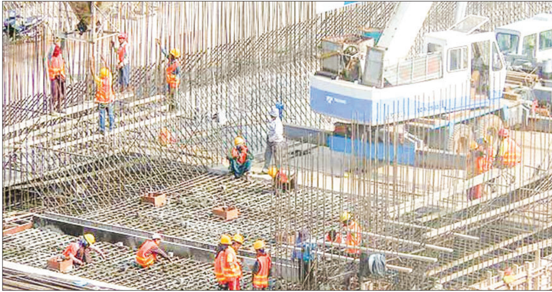
The concrete work for the outlet channel in the Shweli-3 Hydropower Project in Progress.
