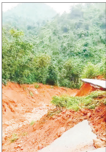
Photos show the collapsed segment of the Asian Highway.
