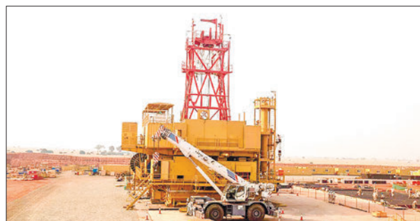
Under construction: An oil well at Murchison Falls National Park in western Uganda, pictured in February this year. PHOTO: BADRU KATUMBA / AFP/FILE
