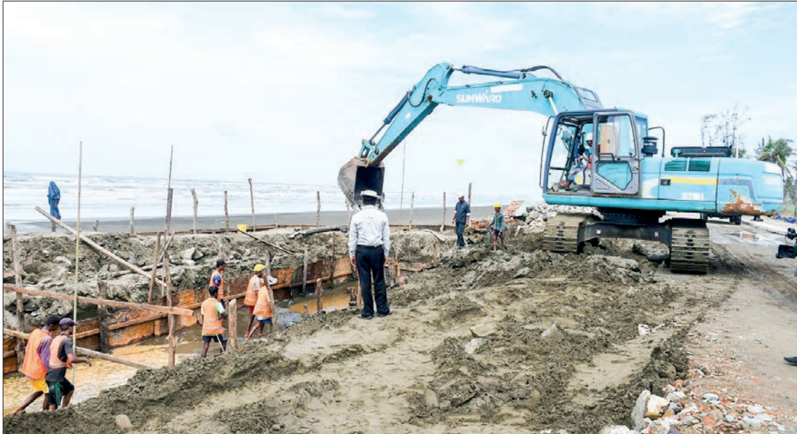
The construction site of expansion of the beach circular road is seen in Sittway on 9 July.
