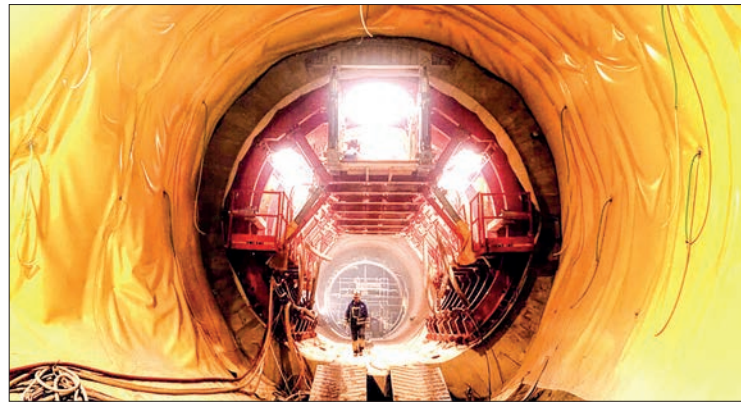
Excavation work for the Limberg 3 pumped storage power plant is wrapping up. PHOTO: JOE KLAMAR / AFP
