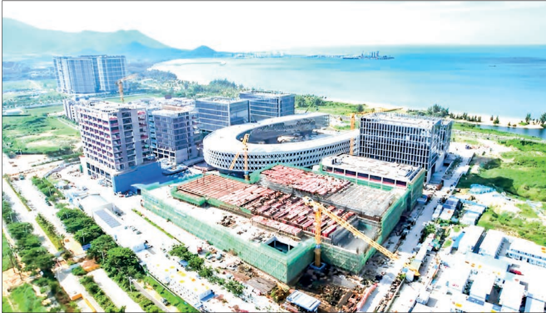
This aerial photo taken on 17 October 2022 shows the construction site of the deep-sea science and technology innovation public platform of Yazhou Bay Science and Technology City in Sanya, south China's Hainan Province. PHOTO: YANG GUANYU/XINHUA
