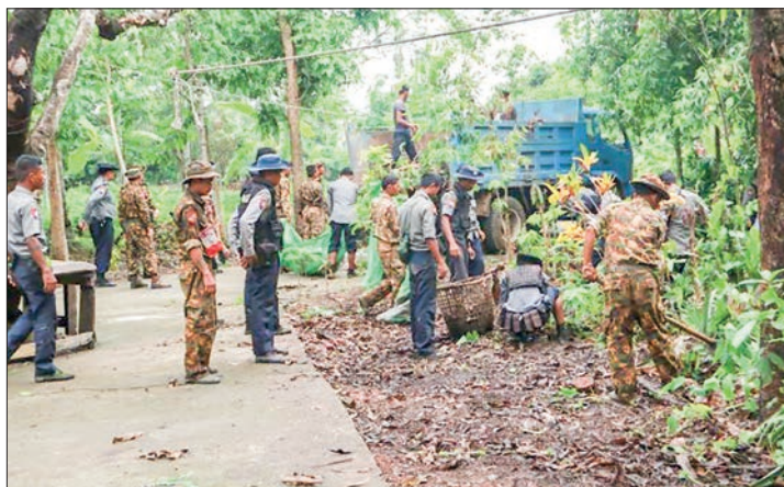
Clear-up measures are underway by relief teams in the Mocha-hit area.
