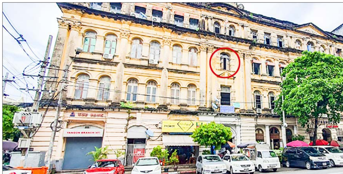
A remote mine blast on the third floor of the Internal Revenue Department office in Yangon on 5 June 2023.
