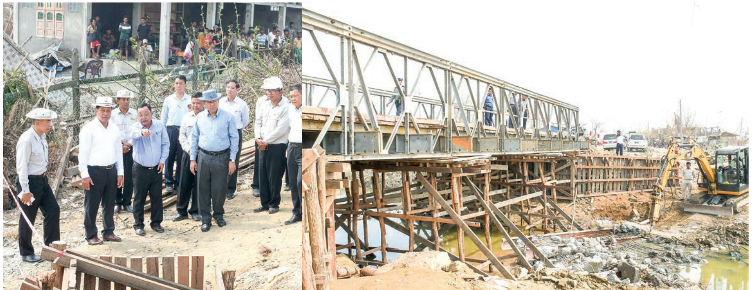
Deputy Prime Minister Admiral Tin Aung San inspects the construction of the Darpaing Bridge in Sittway yesterday.
