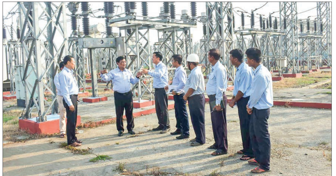
Union Electric Power Minister U Thaung Han inspects the repair and reconstruction works in Rakhine State.
