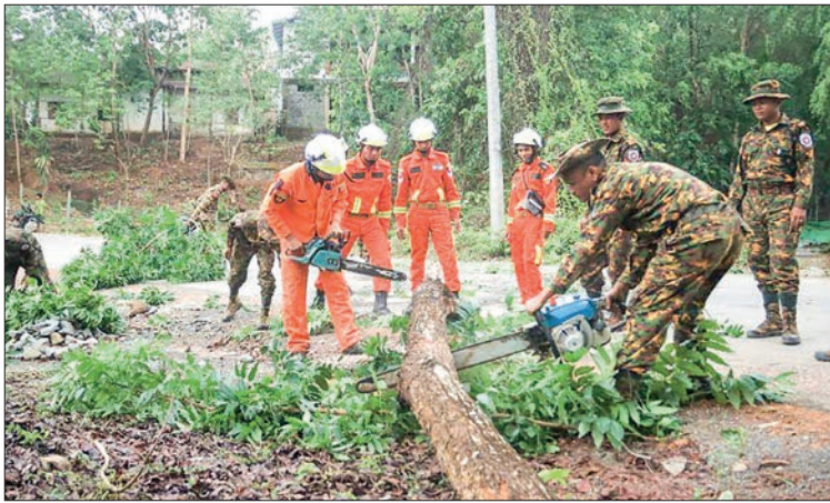
Clearing the fallen trees in Pyintaw village, An Township.
