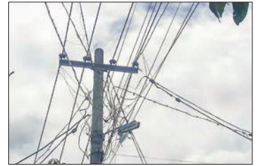
Electric cables connected to the lamp-post.
