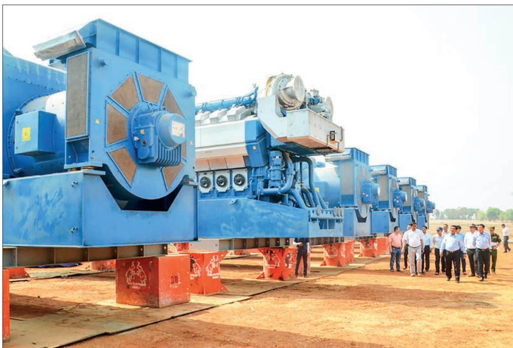
The photo shows solar+gas engine machinery for the hybrid power plant in Magway Township.
