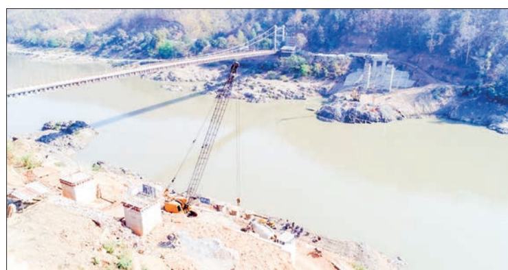
The photo shows the construction of the new Thanlwin Bridge (Tahsan) on the Namhsam-Mongnai-Mongton-Monghsat road. PHOTO: SOE MYINT AUNG
