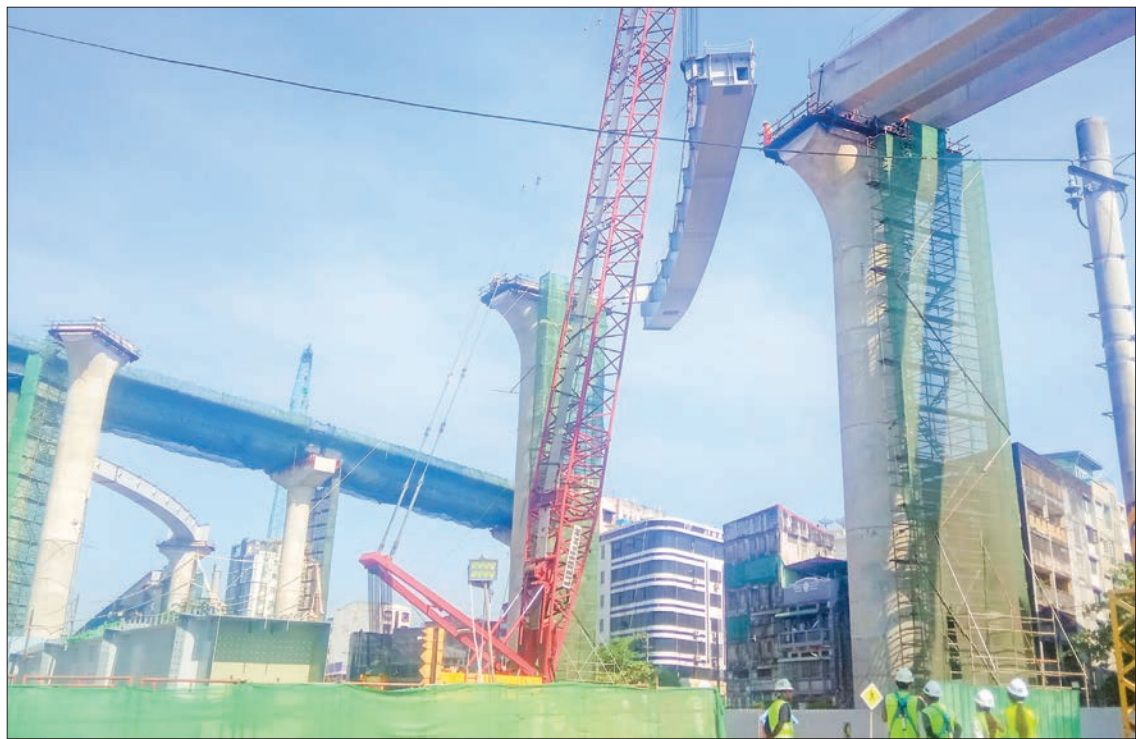
The construction of the Yangon-Dala Bridge is seen from the Yangon side on 23 March 2023. PHOTO: KANU
