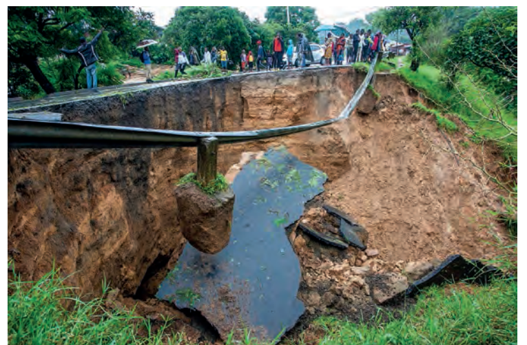
A general view of a collapsed road caused by flooding waters due to heavy rains following cyclone Freddy in Blantyre, Malawi on 13 March 2023. PHOTO: AFP
