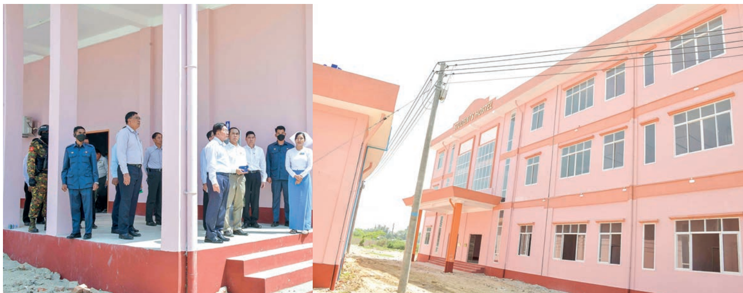
The Senior General views the construction of the new building at the Nursing and Midwifery Training School yesterday.
