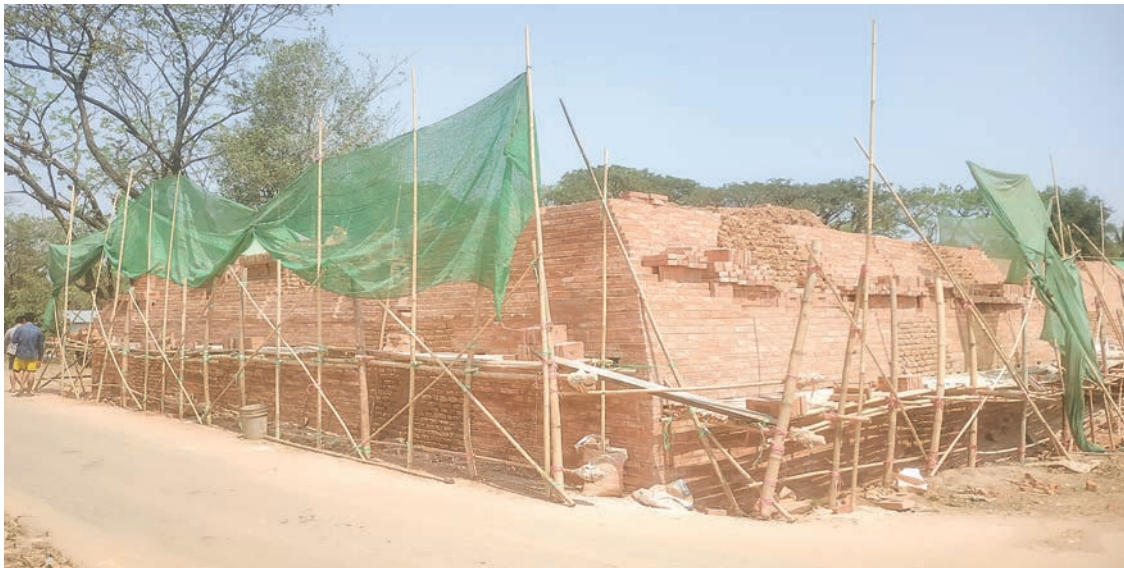
Excavation and reconstruction are underway for the ancient Hanthawady city's southern rampart.
