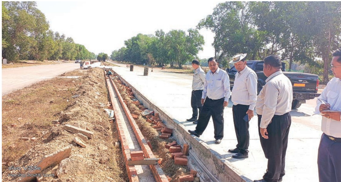
Deputy Minister for Construction U Win Pe and party inspect the drainage system on the Yangon-Mandalay Expressway.
