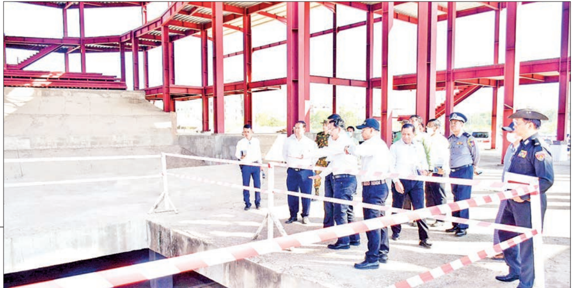
Union Minister U Maung Maung Ohn and Chief Minister U Myo Aung of Mandalay Region views the construction of the Fine Arts Centre (Mandalay) yesterday.
