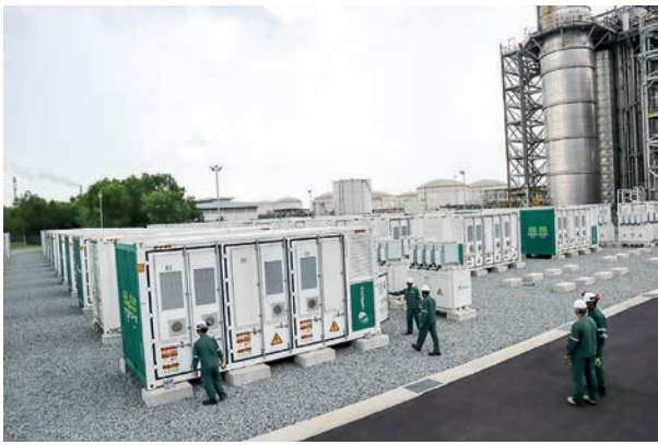
Photo shows workers checking the Sembcorp Energy Storage System on Singapore's Jurong Island on 2 February 2023. PHOTO: KYODO
