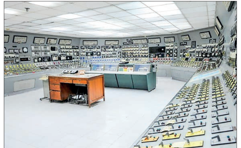
This photo taken on 18 May 2011, shows the main control room of the Bataan Nuclear Power Plant, in Bataan. PHOTO: JAY DIRECTO/AFP/FILE
