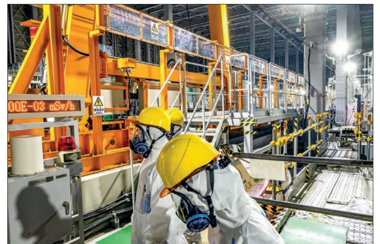
Staff members visit the multi-nuclide removal system of the Tokyo Electric Power Company's (TEPCO) Fukushima Daiichi nuclear power plant, in Okuma of Fukushima prefecture on 20 January 2023. PHOTO: AFP
