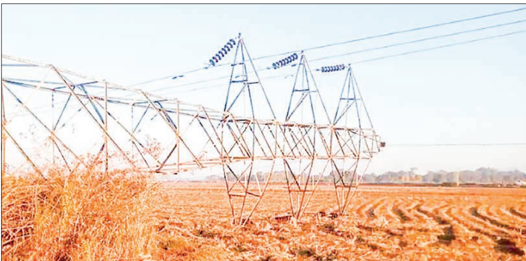
A photo shows fall of tower for 132KV Biluchaung(2)-Tikyit double power cables.
