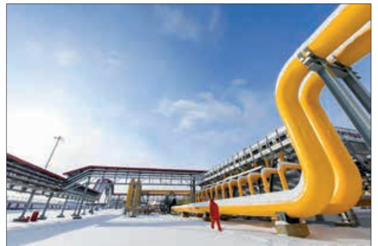
A staff member walks past pipelines in a section of the China-Russia east-route natural gas pipeline in Heihe, northeast China’s Heilongjiang Province, 19 November 2019. PHOTO: XINHUA/WANG JIANWEI/FILE
