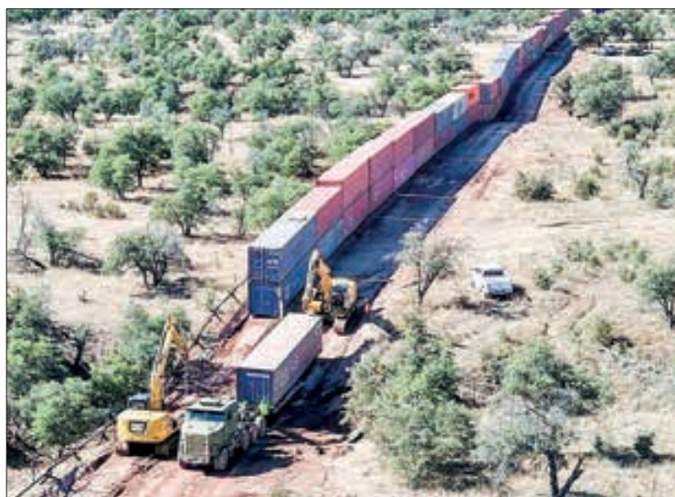
The container wall is being dismantled after being installed just a few months ago at a cost of $100 million to US taxpayers. PHOTO: AFP
