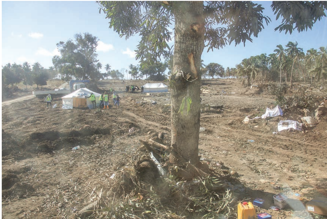
This recent undated handout photo received from the Tonga Red Cross Society on 23 January 2022 shows Red Cross teams setting up temporary shelters in Kanokupolu, a village on the western part of Tonga's main island Tongatapu, after the nearby Hunga Tonga-Hunga Ha'apai volcano erupted on 15 January. PHOTO: HANDOUT / TONGA RED CROSS SOCIETY / AFP
