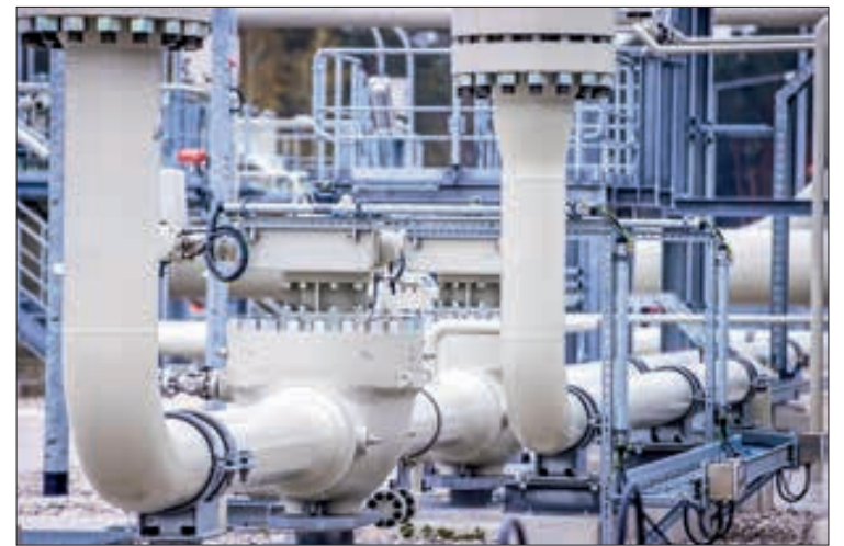
The Nordstream 2 gas pipeline is just one of many casualties of Russia's war in Ukraine. PHOTO: DPA / JENS BUTTNER/AFP
