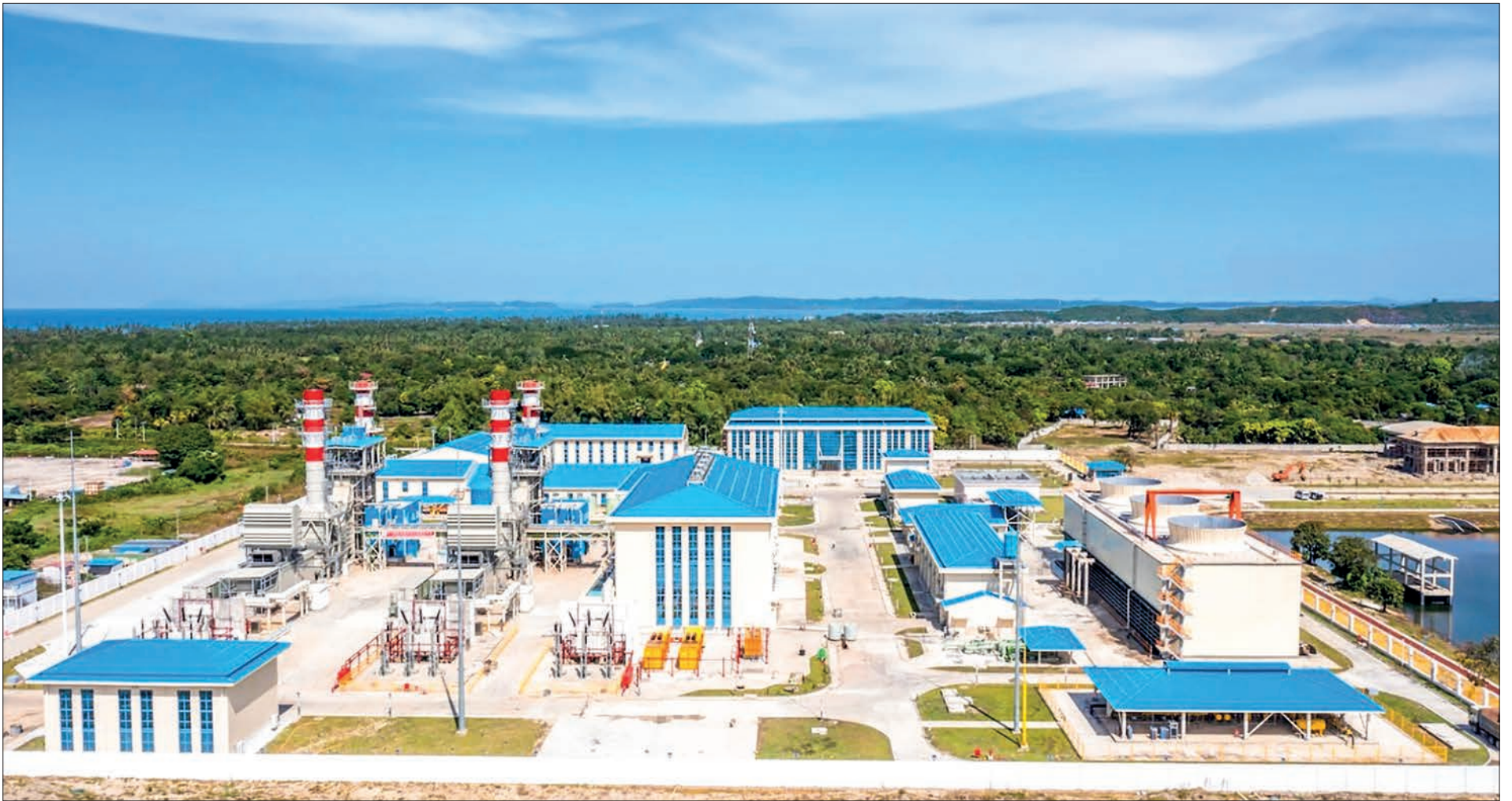
General view of the 135 mW Kyaukpyu combined cycle power plant – one of the FDI projects. The project will be completed in May 2023.
