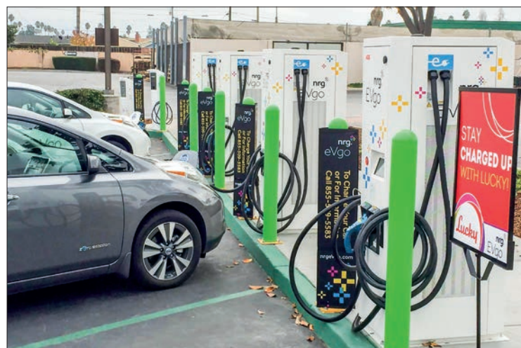
Battery electric cars (BEVs) are seen being charged at the charging station in the foreign country.
