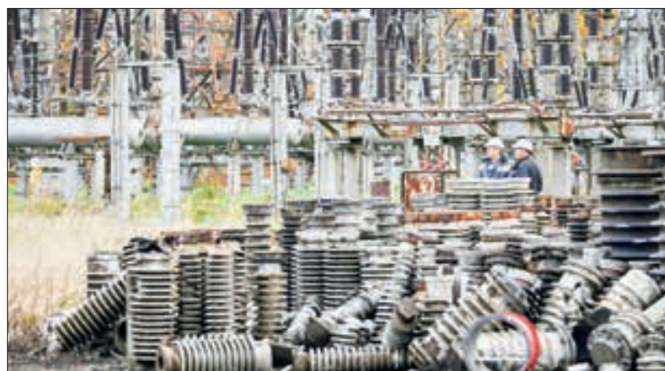
In this file photo taken on 27 October 2022, workers examine damage as they repair power line equipment destroyed after a missile strike on a power plant, in an undisclosed location of Ukraine, amid the Russian invasion of Ukraine. PHOTO: SERGEI SUPINSKY / AFP
