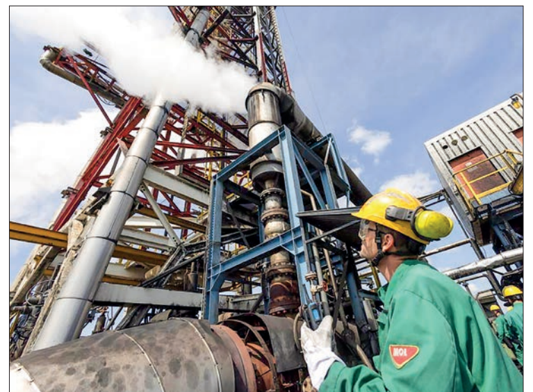
A worker operates machinery at the Danube Refinery in Szazhalombatta, Hungary, 24 May 2022. MOL Group's Danube Refinery is one of the largest refineries in the Central and Eastern European region with a refining capacity of 165,000 barrels per day. PHOTO: ATTILA VOLGYI/XINHUA
