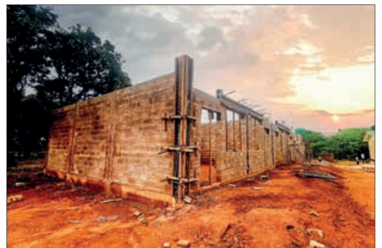
The Masumbu Public Welfare School, built with the assistance of CNMC Deziwa, was under construction on 22 November 2022.
