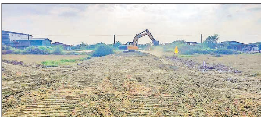
The land for the final disposal site (FDS) project is pictured at the Dagon Myothit (Seikkan) Township.
