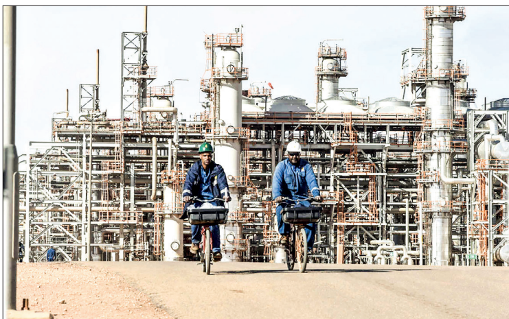
Natural gas processing plant in Amenas, Algeria. PHOTO: RYAD KRAMDI / AFP / FILE
